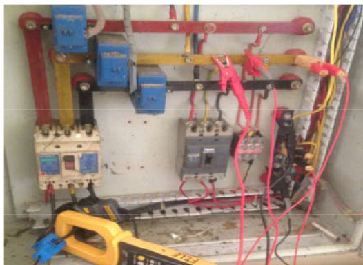
Figure 9(a). Testing wiring procedure of the measurements on the power panel.
